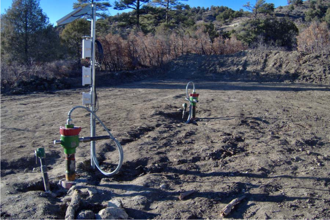
Photo 21: View of telemetry system at the Highway 151 site.
