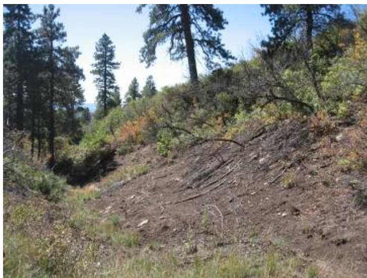
Area of stressed/dead vegetation and methane seepage, text reference VP-1, view south.
