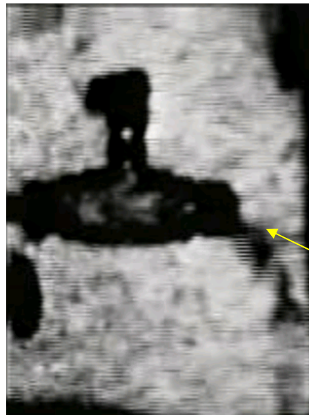
Gas leak at valve using IR imaging
